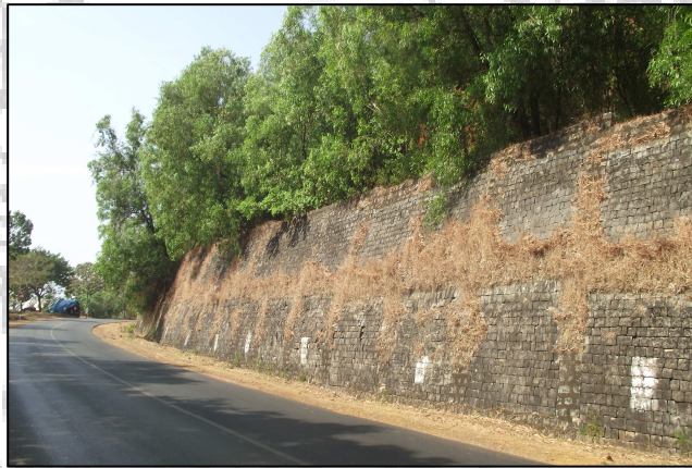
Photo 10: Effective remedial measures in the form of toe wall near facet 67 between Kumta-Ankola
