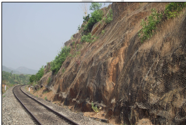
Photo 7: Effective remedial measures adopted by Konkan rail authorities to arrest landslides between Ankola-Karwar.
